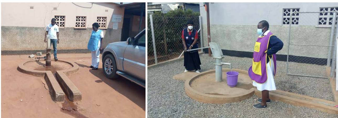
Before and after: This borehole at Mushili Health Centre was non-functional for four years before the SUN TA Project repaired it, restoring access to clean and safe water.
